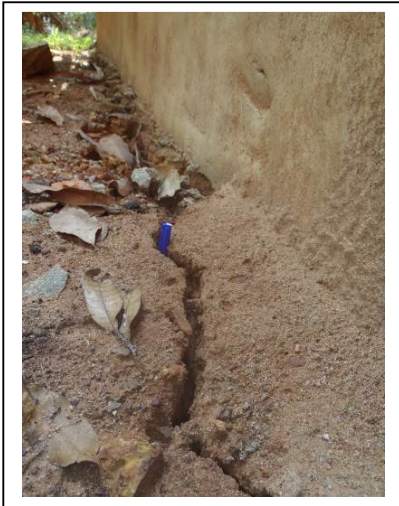
Figure 4: Earth fissures in Vilanthara area
