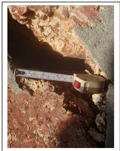
Figure 9: Block separation in the wall cracked
