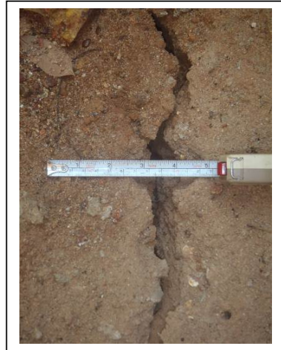
Figure 5: Showing the width of earth fissures (3.5 cm approx.).
