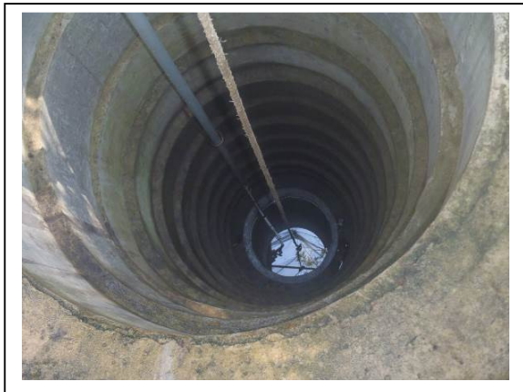
Figure 13: Well with concrete ring collapsed during the land subsidence (Western side of the valley)
