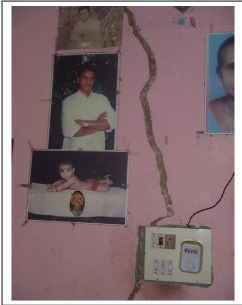
Figure 11: House cracked during the subsidence event
