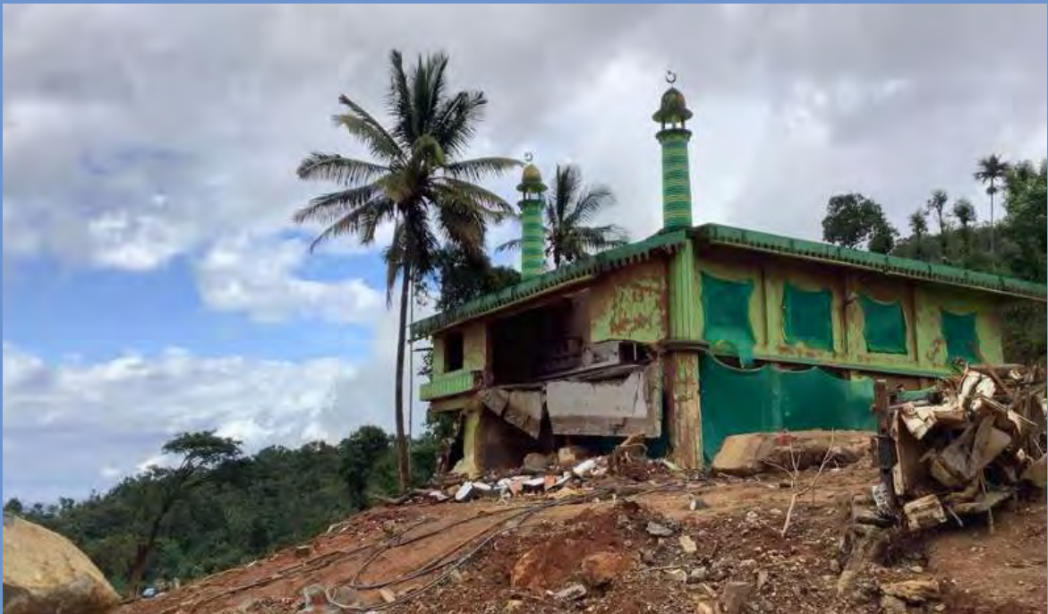
Figure 3-7: Partially damaged Mosque
