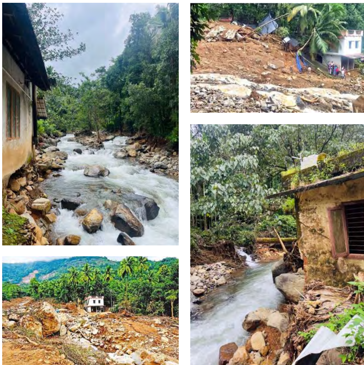
Figure I-3 Housing Damages in Vilangad
