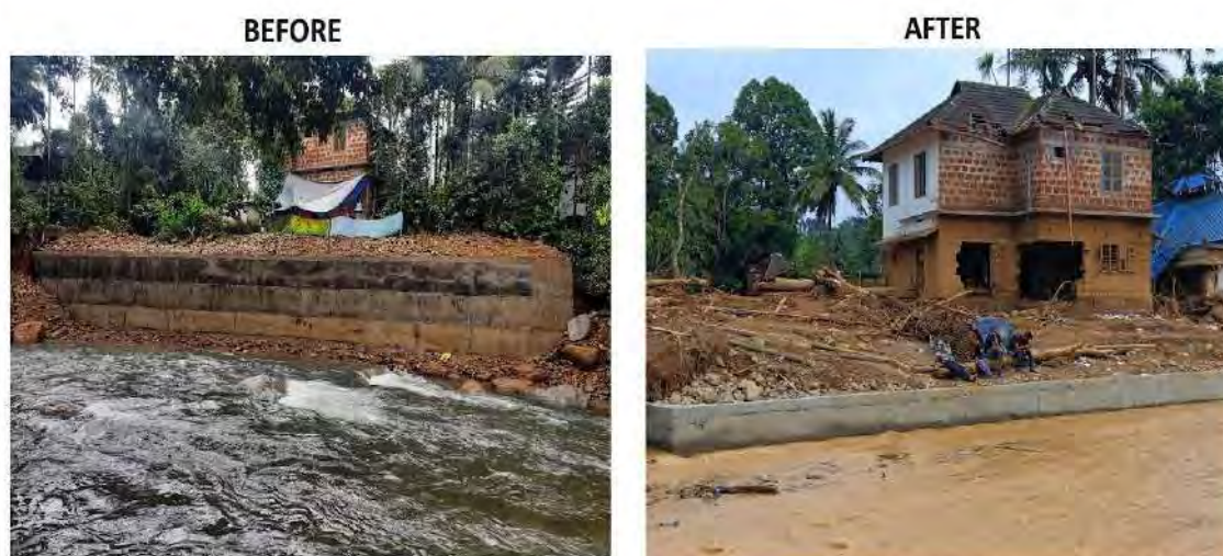
Figure 8-8: Protection wall before and after landslide
