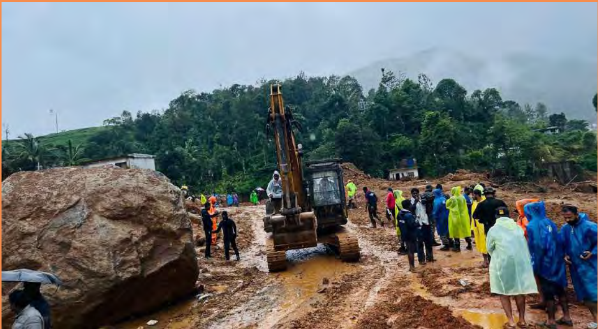
Figure 13-2: Preserve Stone Resort after landslide
