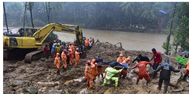
Figure 2-7: Rescue operations carried out at the landslide location near Mackochi in Kokkayar village
