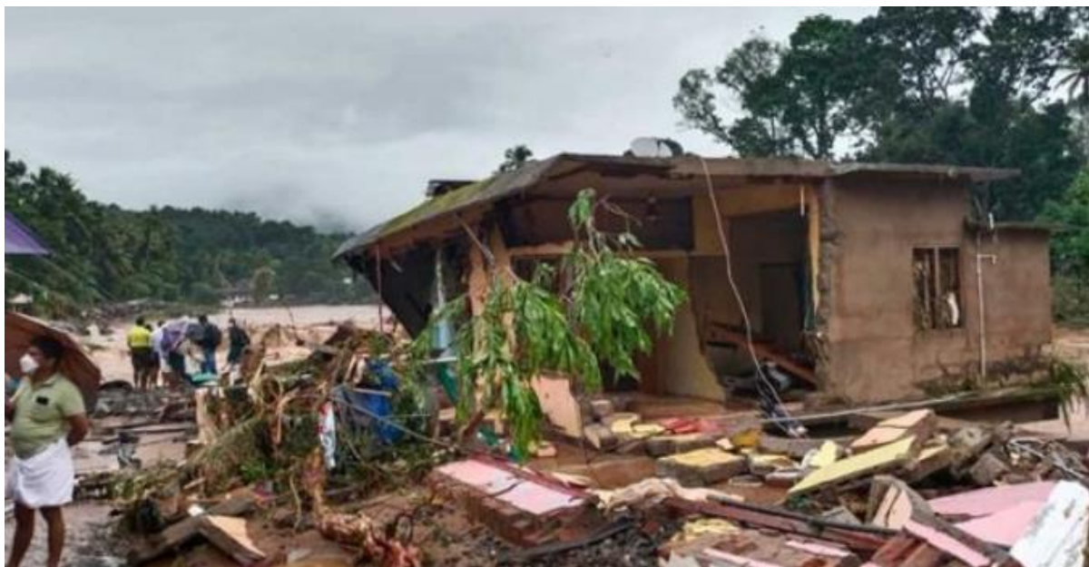
Figure 9-7: Photograph showing a destroyed house at Kootickal
