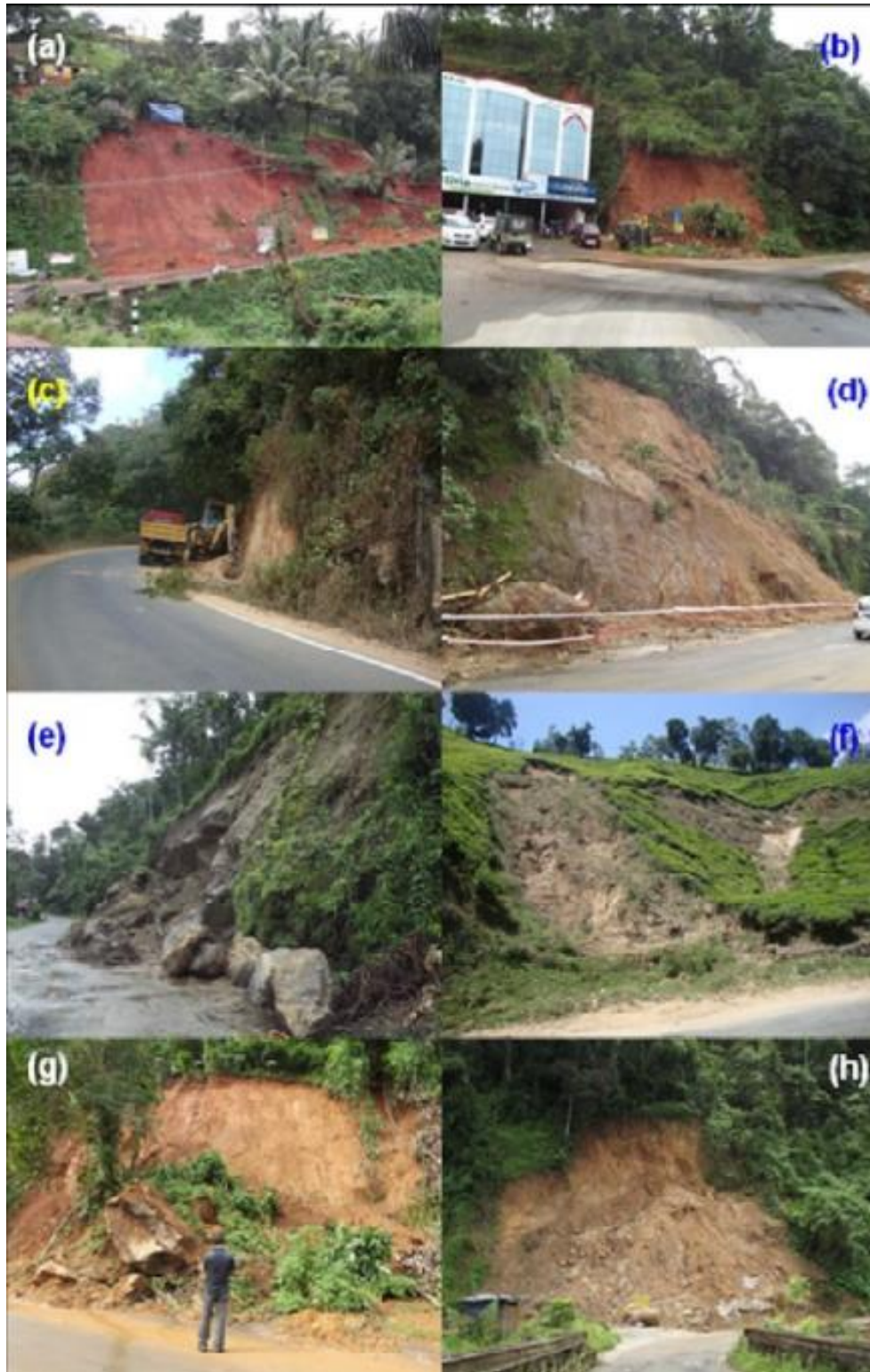
Figure 9-2: Landslides in different parts of Idukki district caused due to the removal of toe for construction of road. a) Cheruthoni, b) Irumbupalam, c) Chinnakanal, d) Cheeyapara, e) Kirithodu, f) Munnar, g) Adimall and h) Kallar (Modified after GIS 2013 report)
