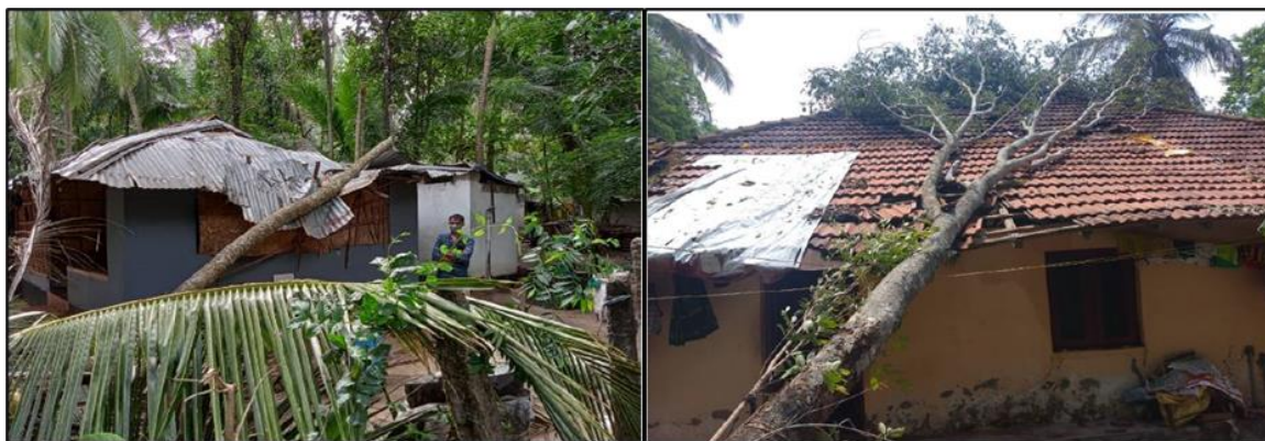
Figure 2-21: House damaged in Malappuram district due to Cyclone Tauktae (Source: District Emergency Operations Centre, Malappuram) (left); House damaged in Palakkad district due to Cyclone Tauktae (Source: District Emergency Operations Centre, Palakkad) (right) (Source: KSDMA)
