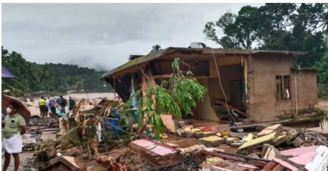
Figure 2-12: Photograph showing a destroyed house at Kootickal
